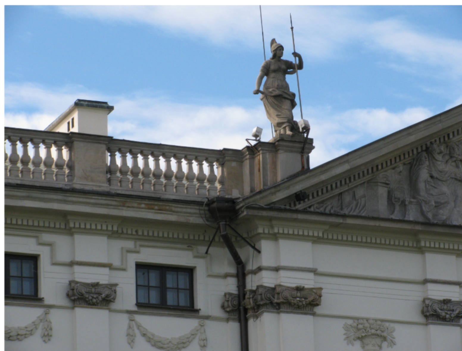
A close-up of the window of the room 218. Behind the drain-pipe there is a wall that showed the water activity. So far the exact reason of the leak has not been discovered yet. Even now in 2013 the wall above the window still "takes the water". The building itself is a monument of heritage and no repairs without the approval of the General Conservator of the Monuments of Heritage can be done.
